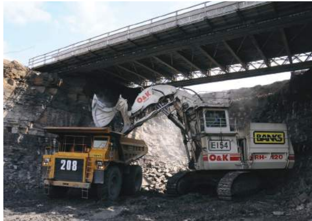
BELOW: The coal areas and the existing compound of the Brenkley Lane Surface Mine were separated by Ponteland Road. To avoid the need to cross the highway we constructed a bridge (with the aid of Cheetham Hill Construction) to support the highway and then excavated the earth underneath to create an access tunnel. BOTTOM: Brownfield remediation at Moss Nook, St Helens
