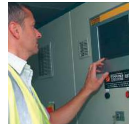
ABOVE/RIGHT: Methane gas collection and electricity generation
