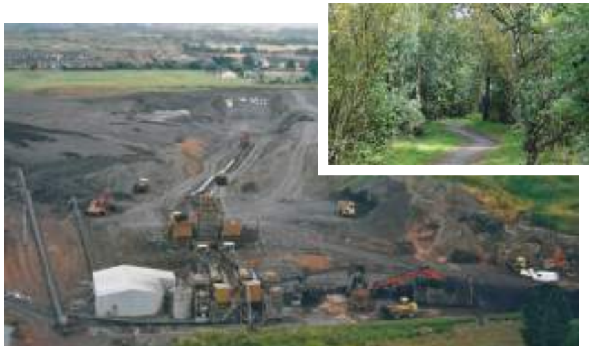
ABOVE: The former Princess Pit at Haydock, St Helens which we reclaimed to create new housing, commercial properties and our first public park, Plele Park (inset)
