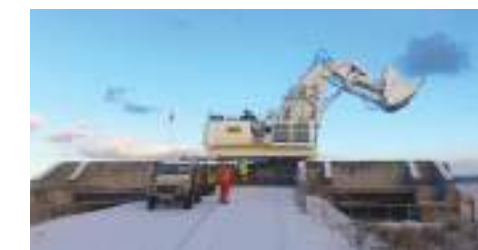
LEFT: Our construction team built a bridge allowing access to the two working areas at the Rusha Surface Mine, which were separated by two large water mains which supply water to the City of Edinburgh
