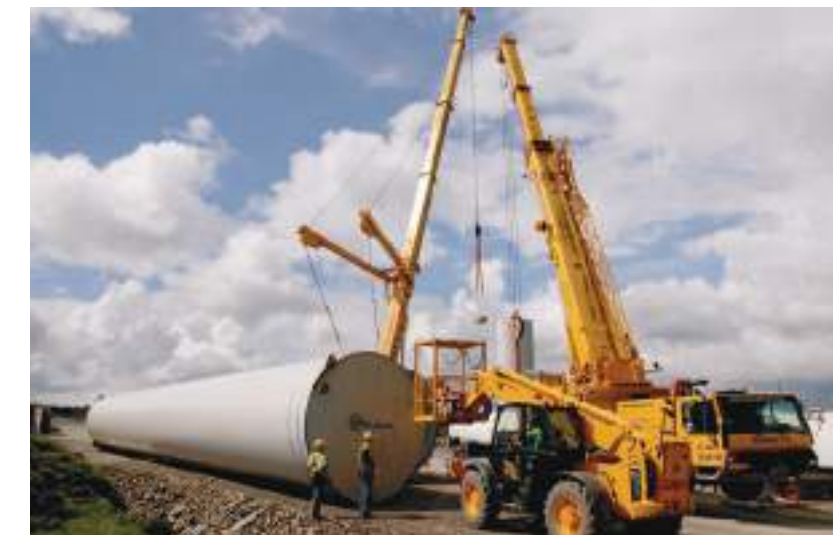
BELOW: Civil engineering at West Durham Wind Farm included creating access tracks and supervising the building of turbine foundations before the turbines could be delivered and erected
